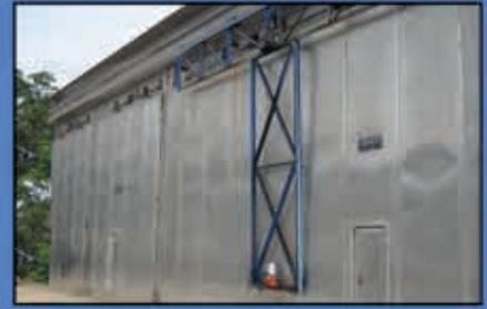
A partial view of the company's dry kilns which have a total capacity of 1,000,000'.
